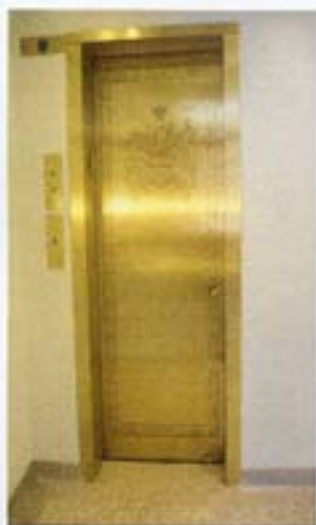
Elevator door with bullet holes.
